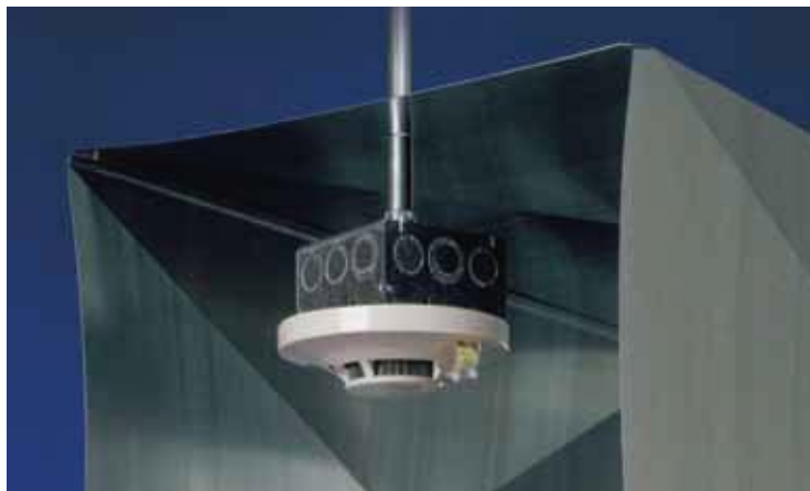
Top Mount in Ventilation Shaft
